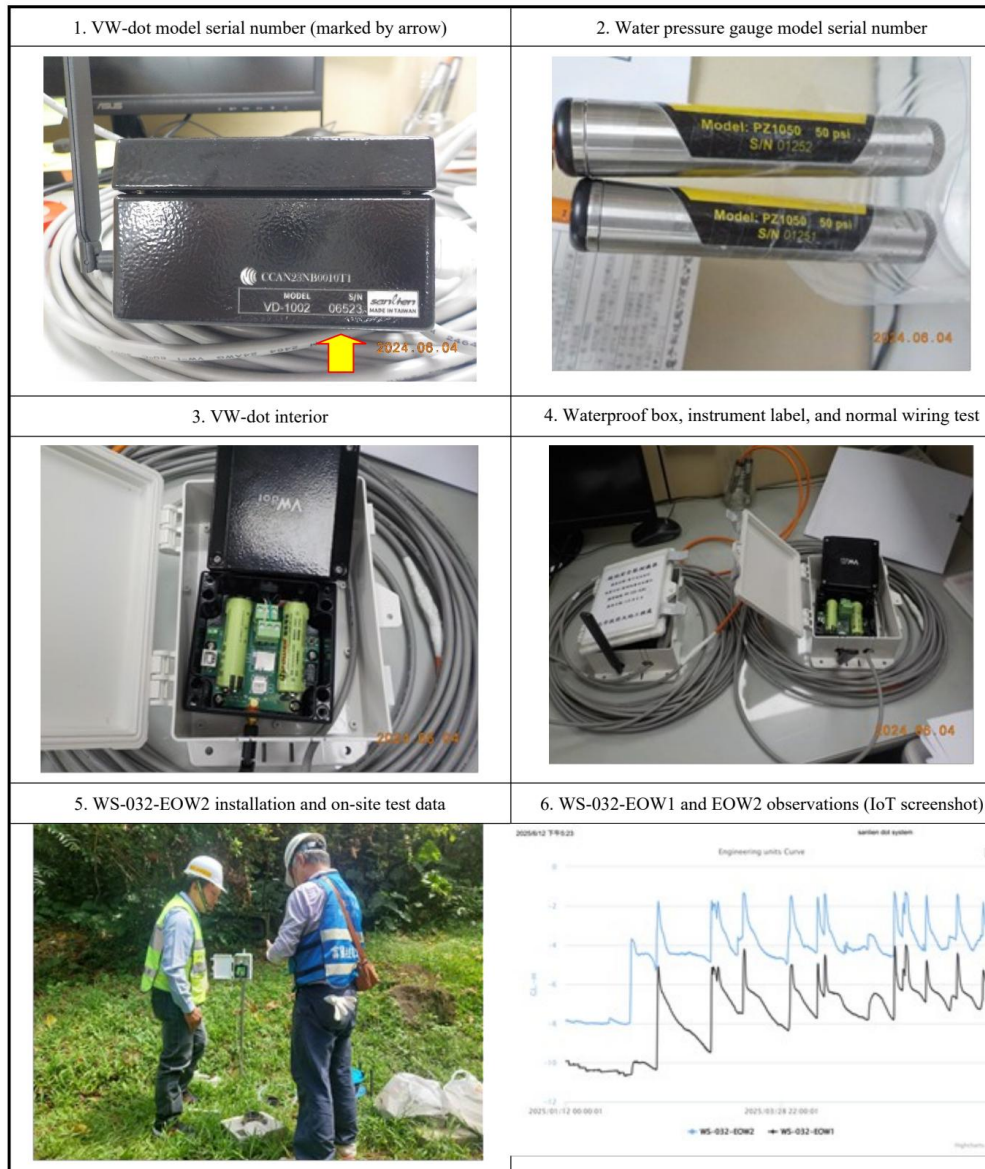
Figure 4. VW-dot and electronic water level observation well automatic recording installation (WS-032 slope).
