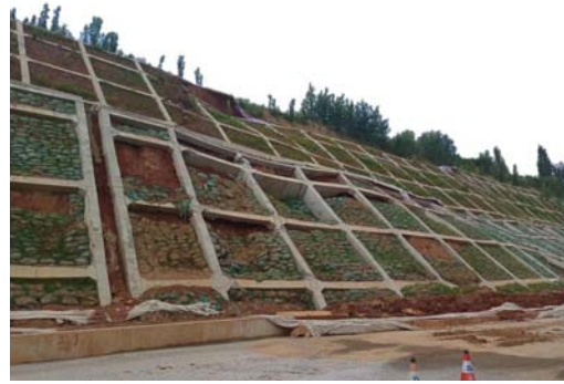
(b) Lixi highway landslide
