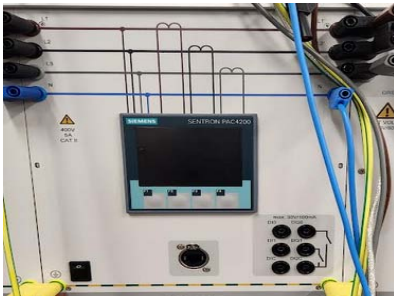
(g) Power Quality Meter
